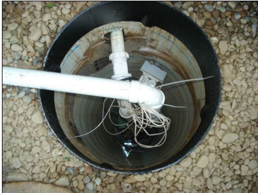
Two discharge lines in crock
