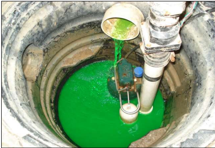
Dye water from a compromised downspout leader flowing into sump pump crock
